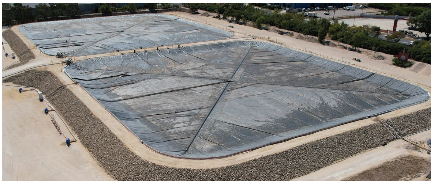
Locally manufactured UAN has already started flowing into the new storage facility at the Kwinana Depot in preparation for the 2024 season.
